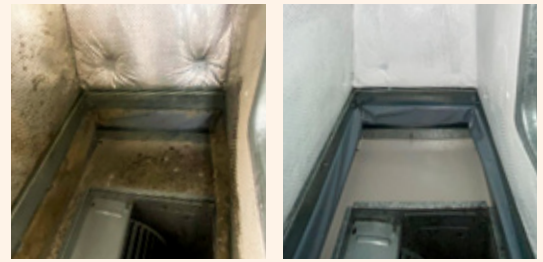
▲ Before & After: A visibly cleaner air conditioning unit following professional decontamination.
